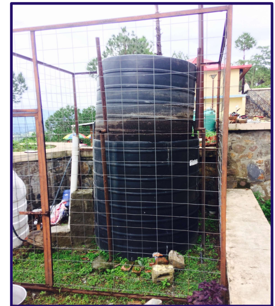
Biogas Reactor at Jaypee University, Solan VID-20191128-WA0002.mp4
