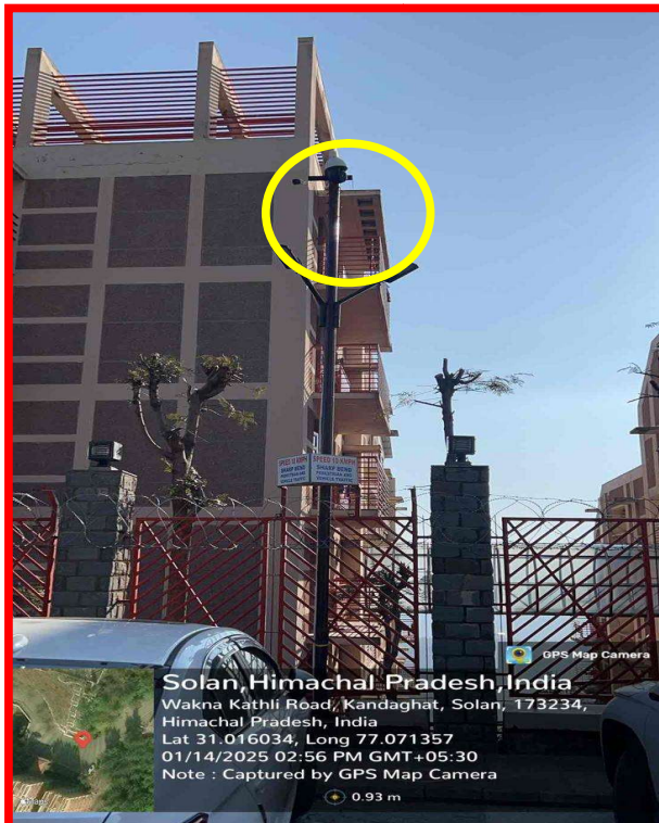
Fig 4: CCTV camera installed in front of
